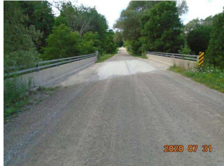
Images of Bridge in Poor Condition Nature Center Road Bridge
